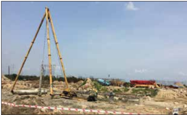
RFL HDPE Water Distribution Line at Modunaghat Water Treatment Plant, Chittagong
