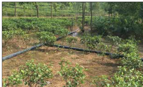
RFL HDPE Pipe Line at Tea Garden, Chittagong
