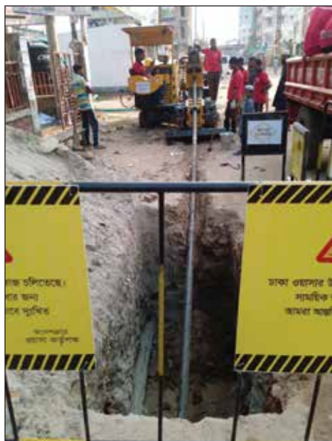
RFL HDPE Potable Water Line, DWASA ICB02.7 Package
